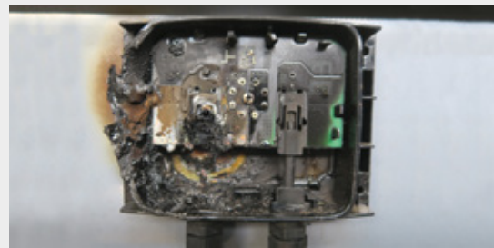
Figure 2: Burned wall socket due to corroded contacts
