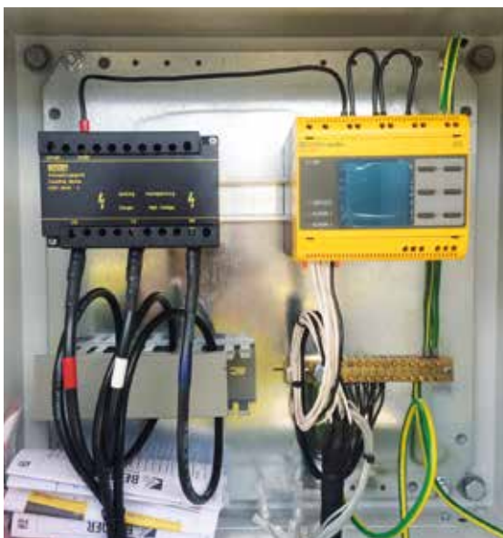
iso685-D installed on the wellhead
