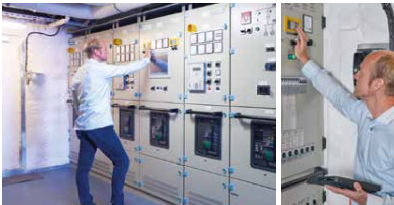
Function check – Benjamin Greiff checks the insulation monitoring system
