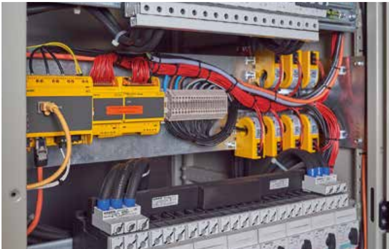
Measuring current transformers are important components for real-time insulation fault location © Carsten Müller
