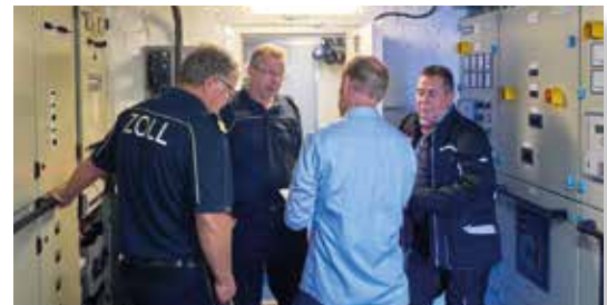
Discussion about the insulation fault monitoring system © Carsten Müller
