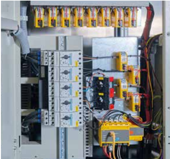
440 V machine network monitoring with the assignment of insulation faults to the exact output © Carsten Müller
