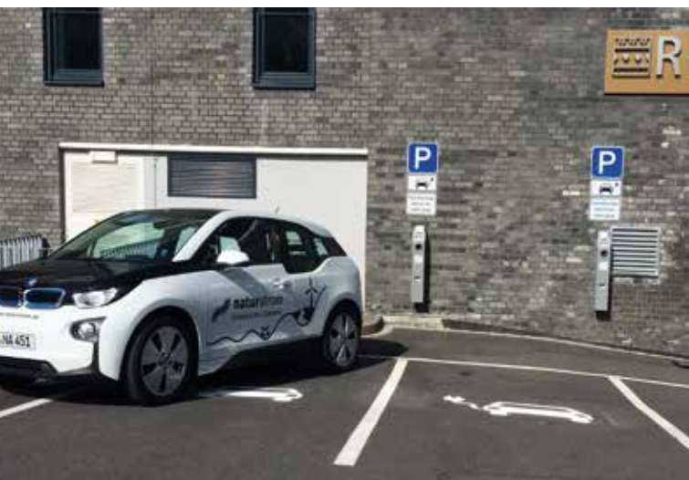
Figure 2: Since 22 July 2019, the Cologne City Hotel has been operating two wallboxes from the Bender subsidiary ebee that comply with German calibration law. The 100 % green electricity used here is supplied by NATURSTROM AG.
