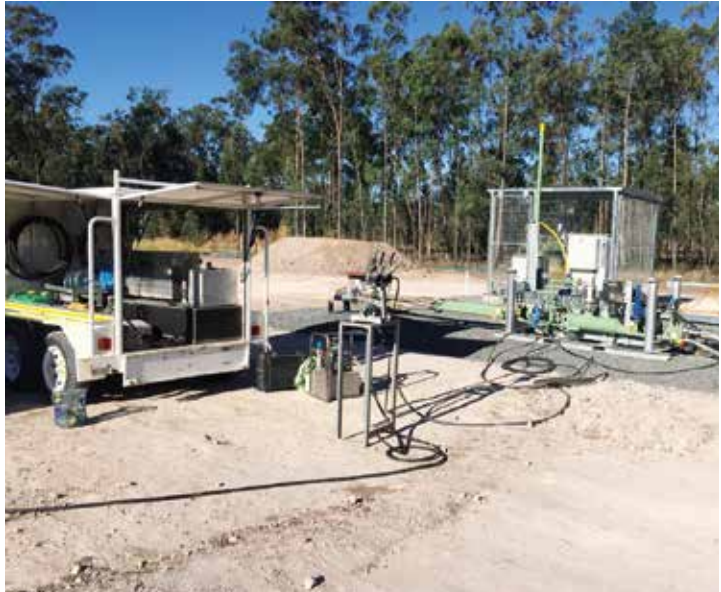
Wellhead during commissioning
